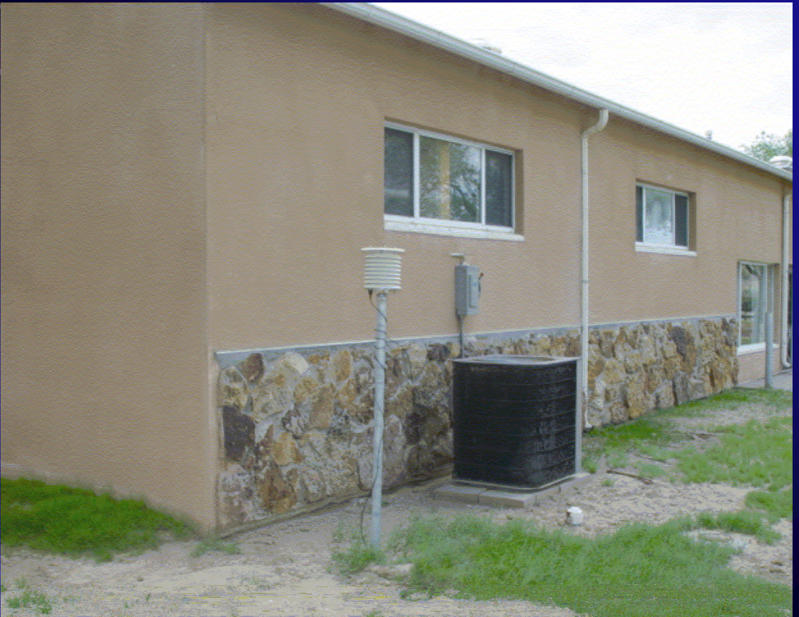
MMTS installation near John Martin Reservoir, Colorado.
