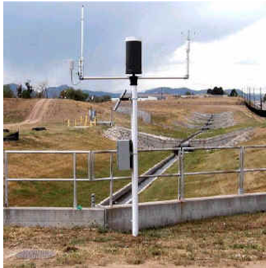
New ALERT weather station & stream gauge on Marston Lake North Drainageway.
